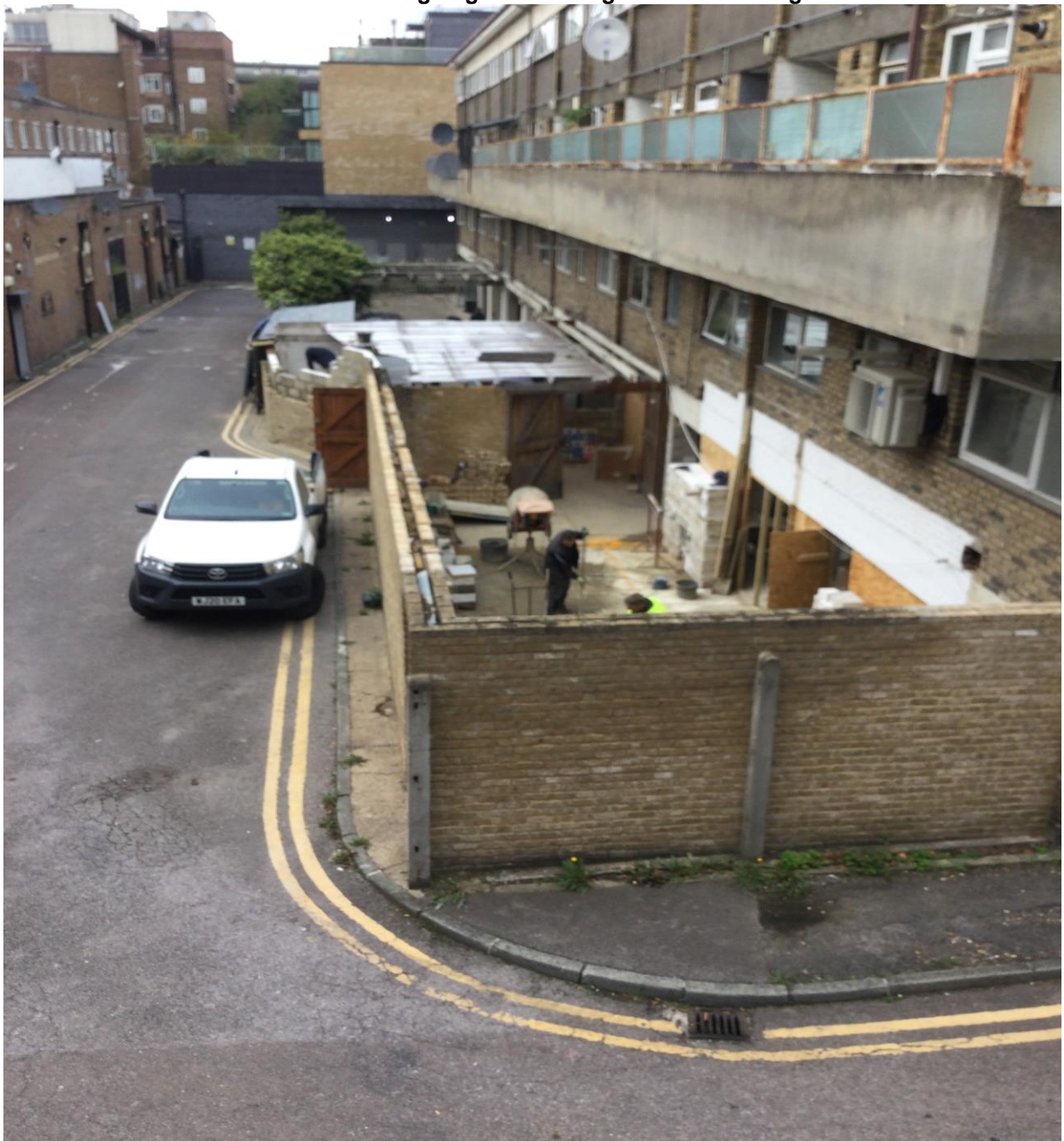
Rear elevation of Cervantes Court – garages at lower ground level being converted into 2 flats
